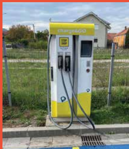
Stop Shop Čačak punjač snage 120 kW
